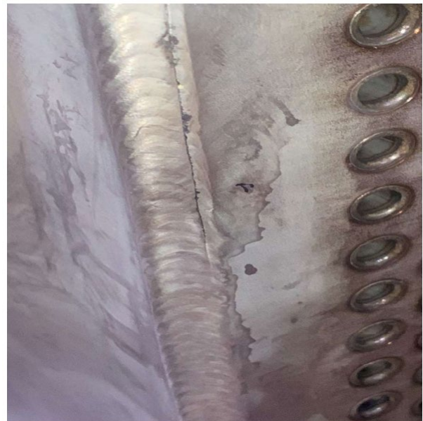
Close-up of cracked weld
